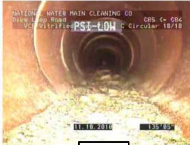
Photo 3: Example debris (CB5->CB4) section of full length of pipe.
