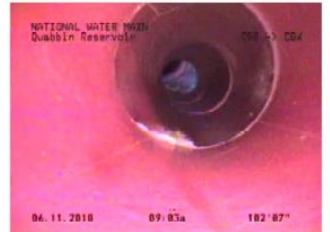
Photo 6: Example concrete deposit/mortar protruding from joint.
