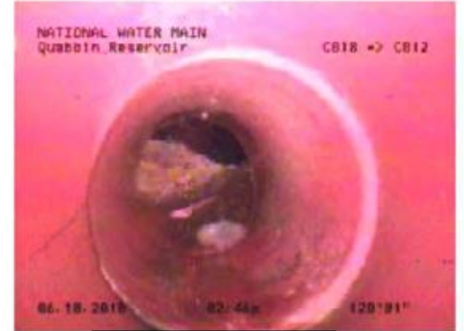
Photo 5: Concrete debris in pipe CB18->CB12.
